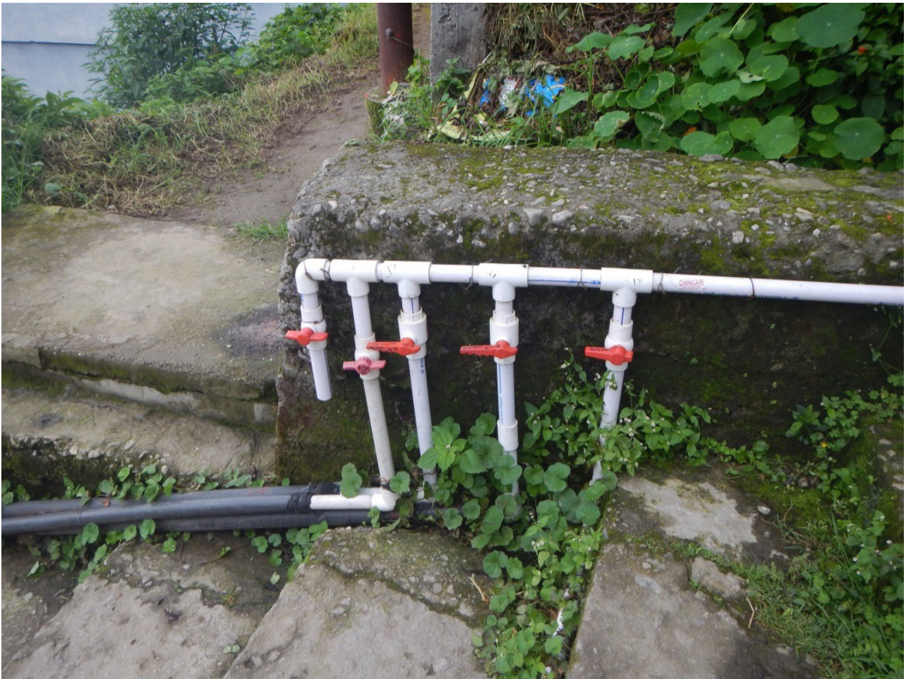
Figure 3: Water Distribution Infrastructure in Frymal Village (Author 2018)
