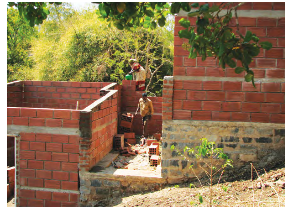
Construction of ATREE's field station in the Biligiri Hills, Karnataka © Mathivanan M
